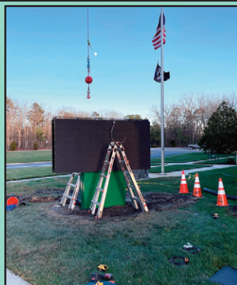
New Digital Sign Installed at Townhall
